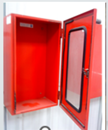
Fire Extinguisher Cabinet
